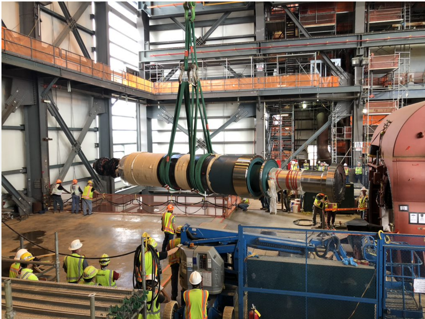
Unit 3 Generator Rotor
