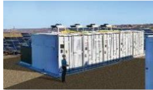
Horn Rapids Solar, Storage & Training Project (4 MW)
