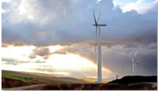
Nine Canyon Wind Project (96 MW)
